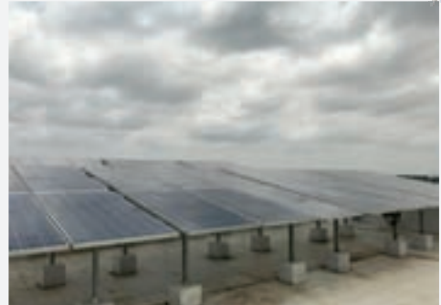
Solar Power Plant of NACIN Bengaluru, the first "Green Building" of CBIC.
