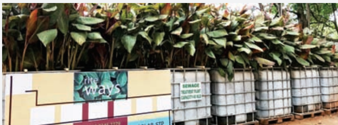
NACIN, Bengaluru installed a sewage treatment plant in its premises
