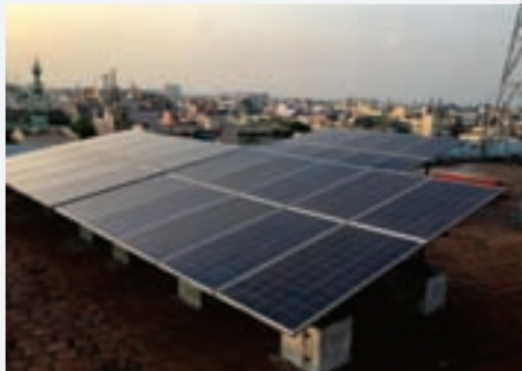
Solar Power Plant installed by Chennai Customs
