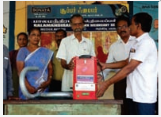
Chennai Appeals II has installed a RO water purifier, in the second floor of Adi Dravida Welfare Govt. Higher Secondary School in Chennai.
